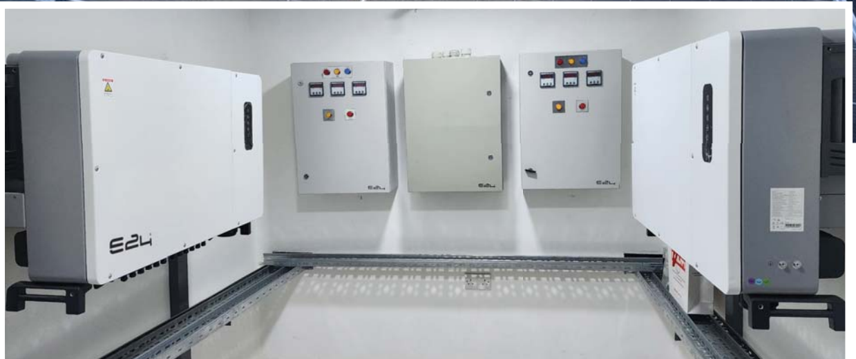
PVISU3-350K powering a university in Nigeria
