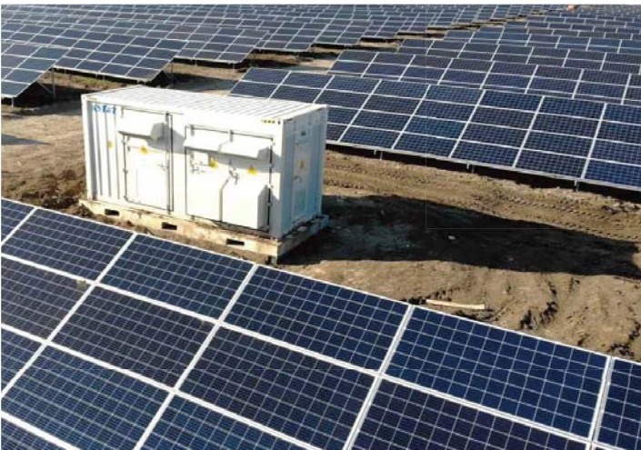
Utility Scale Power Plant of 200MW in Ukraine
