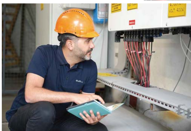
8 units of PVISU3-125KI powering a furniture factory in Turkey (900KW)
